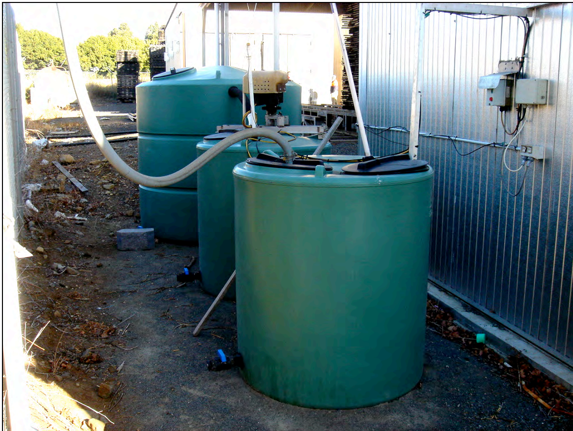
Plate 5: Three-stage treatment system for treating water condensate effluent associated with the timber kiln drying operation.
