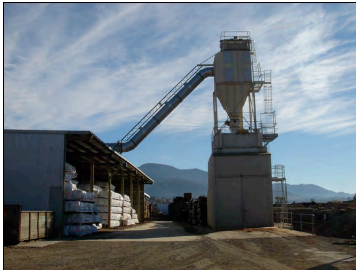
Plate 3: Dry shavings air filtration system and containment, storage and loading hopper.
